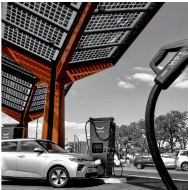
Charging stations for electric vehicles on the A6, Dracé © Erolf production
