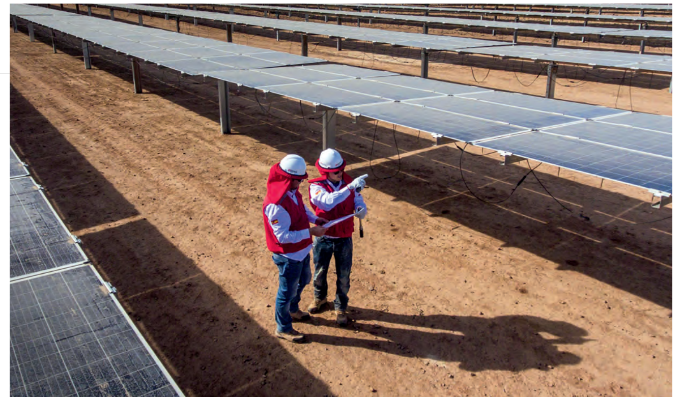
Huatacondo (Chile) — In 2018, our teams completed work on the 103 MWp Huatacondo photovoltaic power plant.
