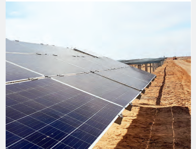
The Huatacondo power plant in Chile has 300,000 solar panels and a capacity of 98 MWp.
