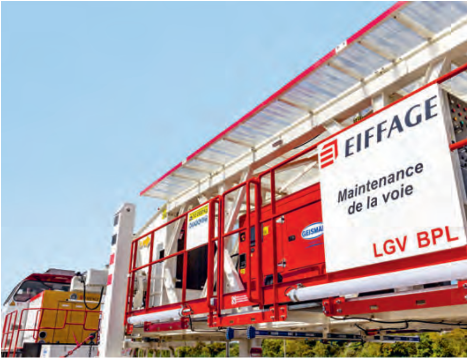
4 Track maintenance train on the Bretagne-Pays de la Loire high-speed rail link.
