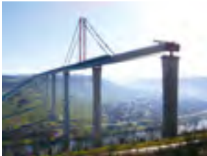
Rhineland-Palatinate (Germany) — The Hochmosel bridge over the river Moselle will be one of the largest steel viaducts ever built in Germany (measuring 1,700 m in length and standing 150 m tall).
