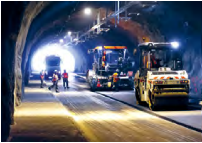
Le Freney-d’Oisans — The Chambon tunnel, which had been closed since 2015 due to a landslide, reopened to traffic in December 2017.
