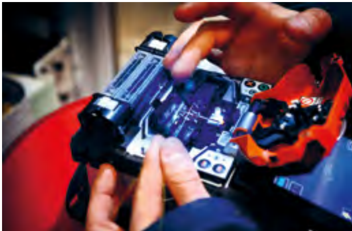
Connecting an optical fibre.
